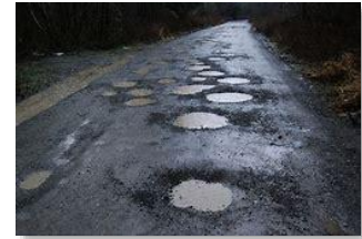
Potholes are smaller.
